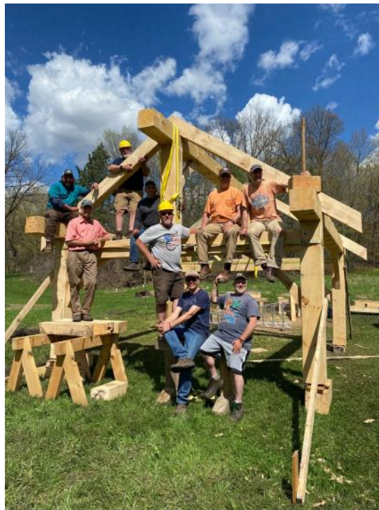
This structure was built by the 2022 class, and it now resides on the Lake Wobegon Trail in Albany. It's a bike shelter.
